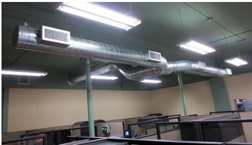
All ductwork is custom fabricated and insulated where necessary
